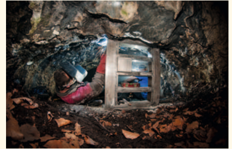
Gate installation in Zbójnicka cave. Construction work in such conditions is not easy.
