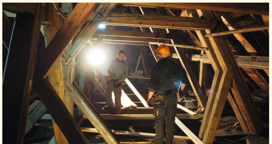
Contractors assembling guano platforms in Górkki Wielkie church – occupied by 300 greater mouse-eared and close to 100 horseshoe bats.
