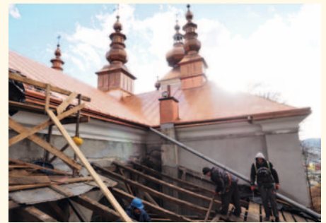
Roof renovation of a Greek Orthodox church in Krynica Zdrój. Winter conditions were challenging for workers.
